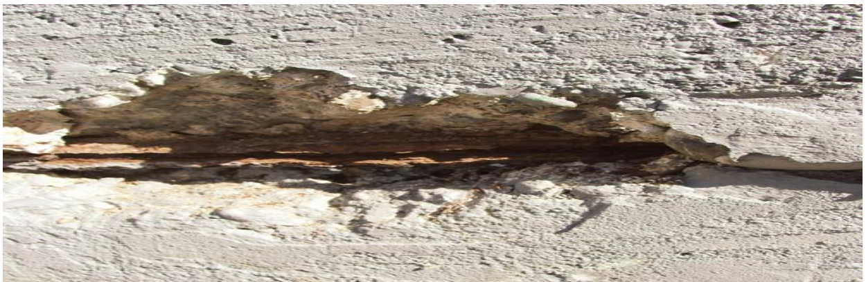
Fig 3 : Spalling due to rusting rebar.
